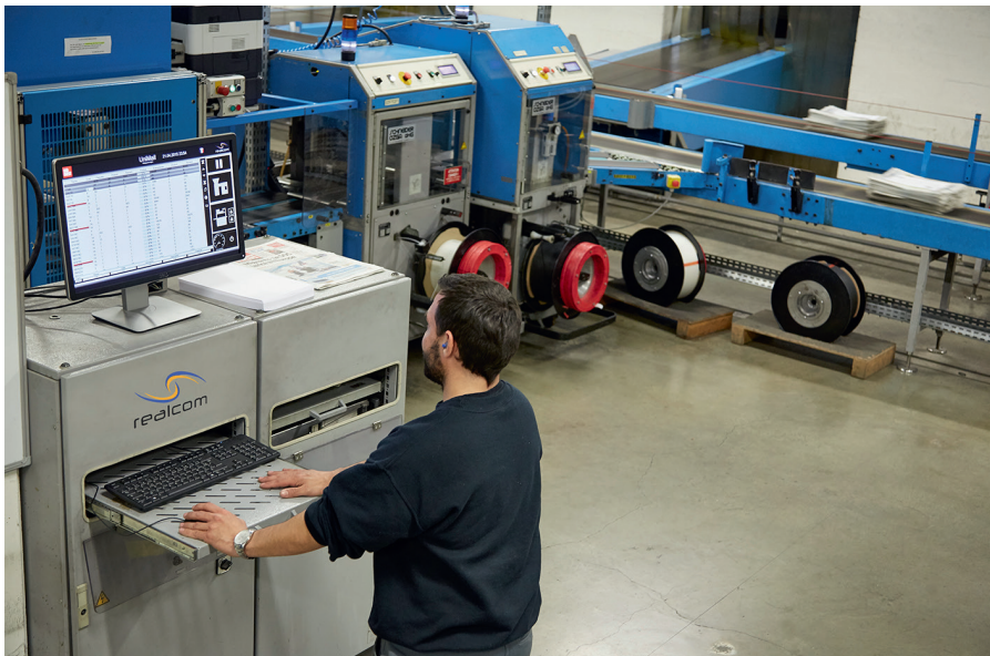
Colour codes make for rapid identification of the different operating conditions for all components in the mailroom system.
